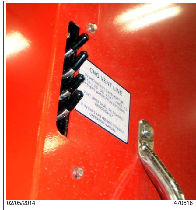
Fig. 21.8, CNG Vent Line Caps
